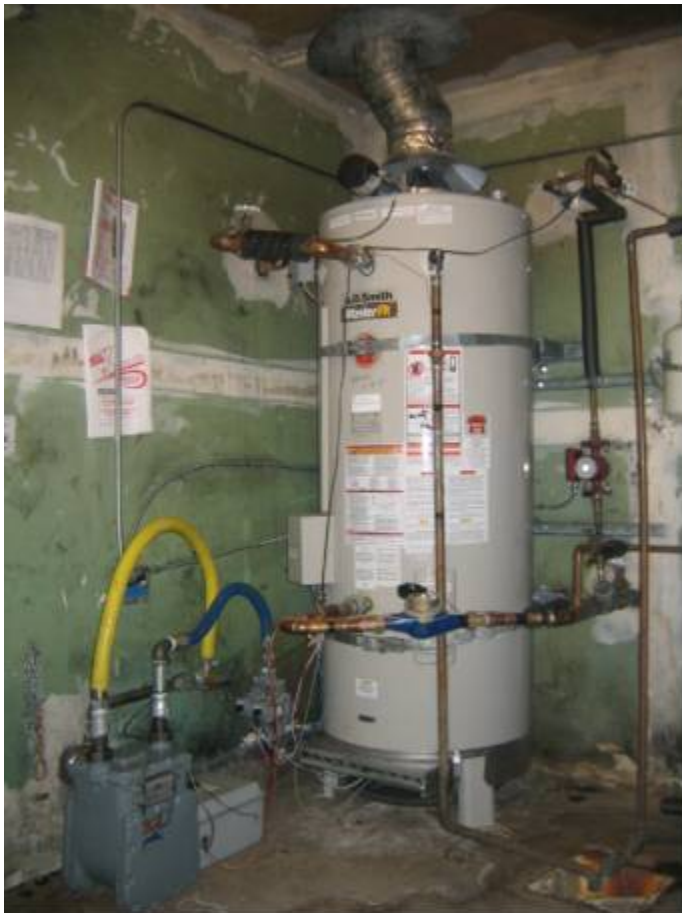
Figure 1. Water Heater in FSR #1 – Dublin, CA
