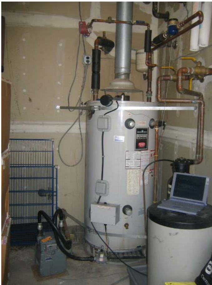
Figure 5. Water Heater in FSR #2 – San Ramon, CA
