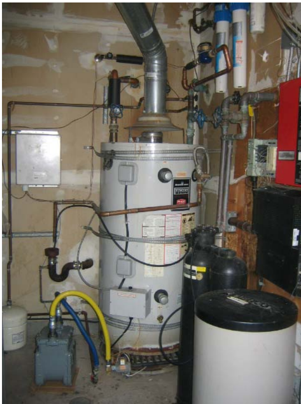
Figure 9. Water Heater FSR #3 – San Ramon, CA
