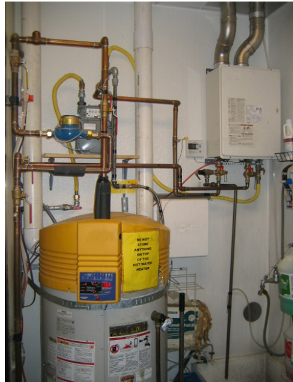
Figure 2. Water Heater Test Arrangement
