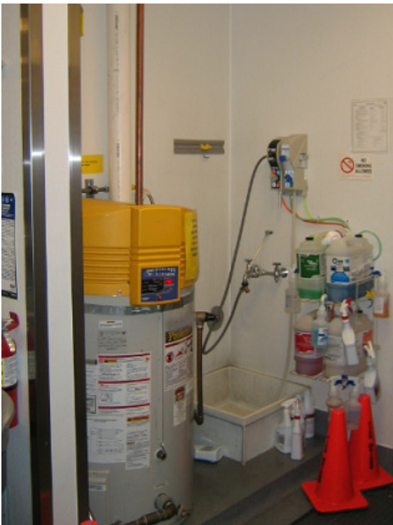
Figure 1. Water Heater as Originally Installed
