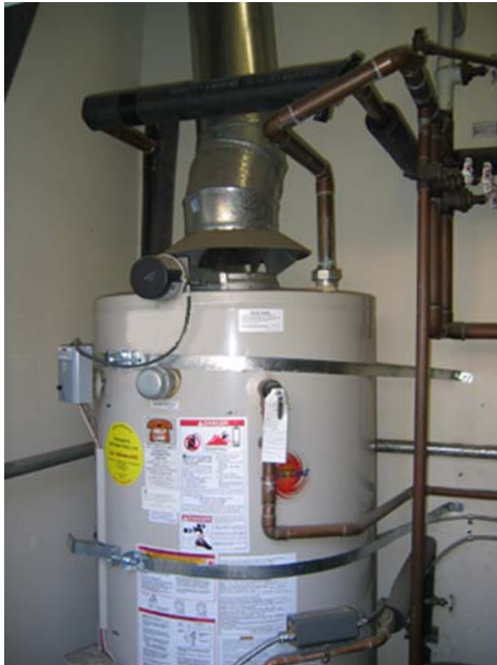
Figure 2. Standard efficiency tank as originally installed
