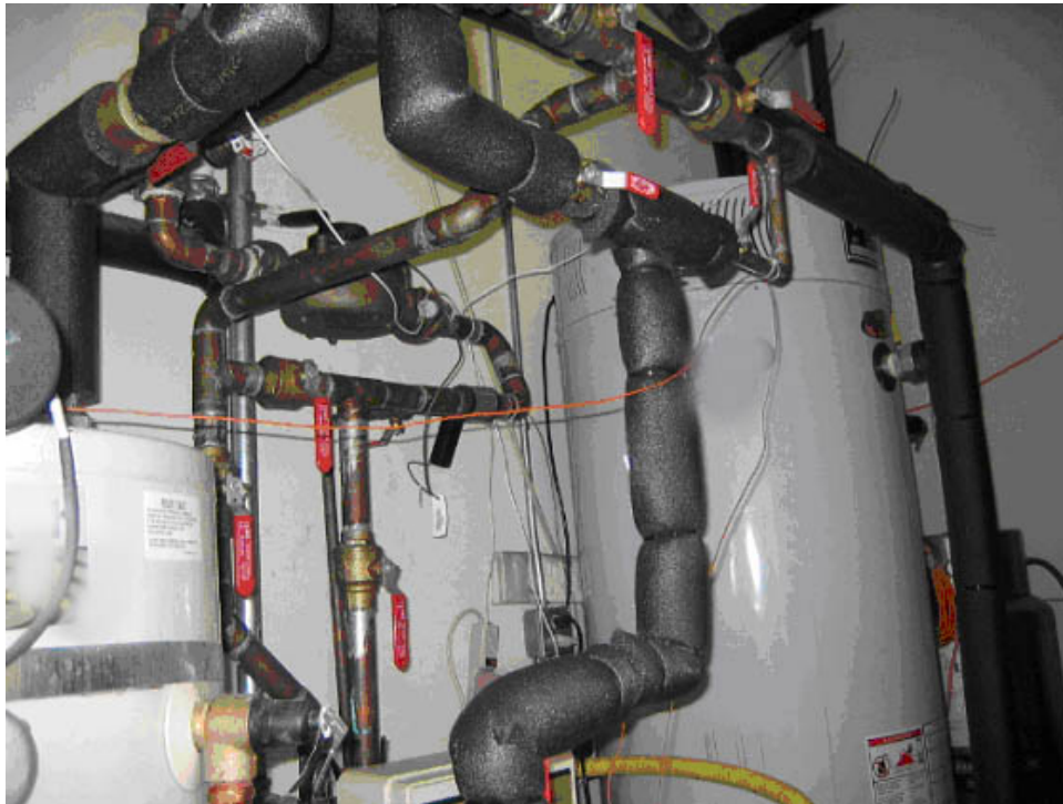
Figure 4. Water heaters installed for monitoring
