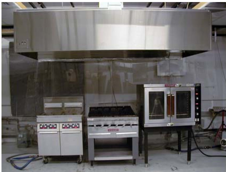
Figure 9. Fryer/Broiler/Convection Oven Appliance Line
