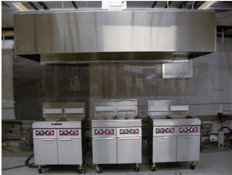
Figure 7. Medium-Duty Gas Fryer Line
