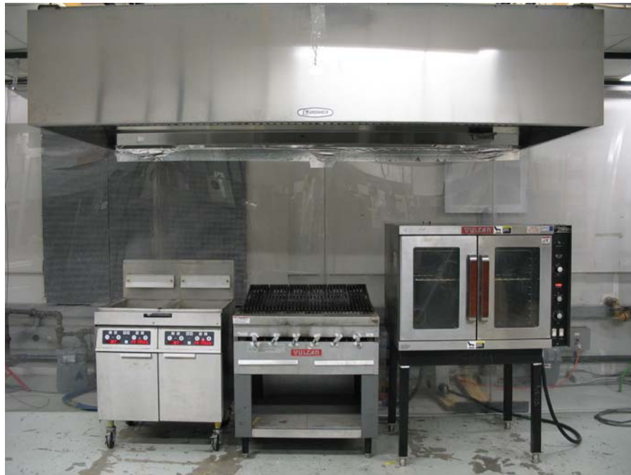
Figure 10. Fryer/Broiler/Convection Oven Appliance Line
