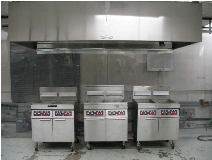
Figure 8. Medium-Duty Gas Fryer Line
