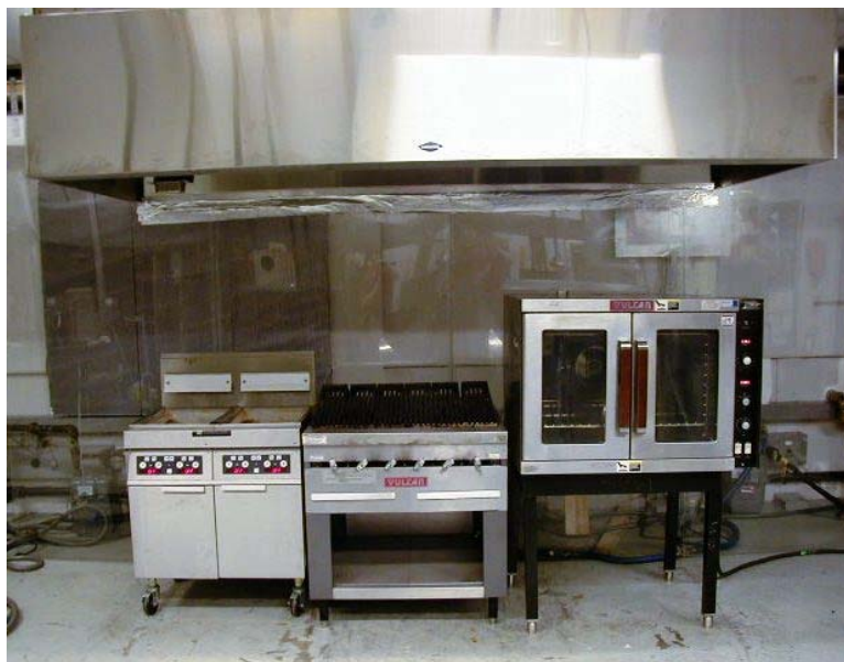
Figure 8. Fryer/Charbroiler/Convection Oven Appliance Line
