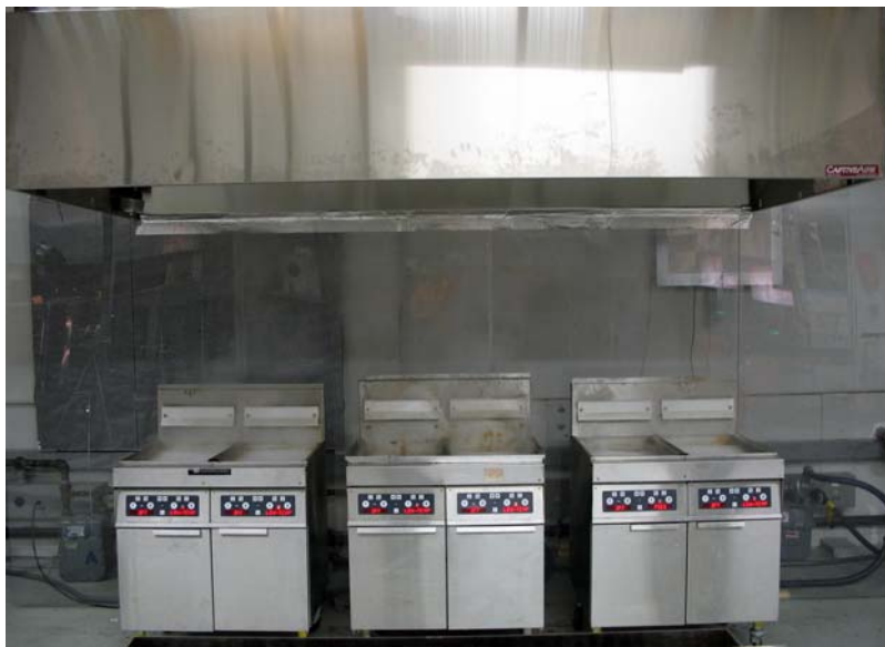
Figure 6. Medium-Duty Gas Fryer Line
