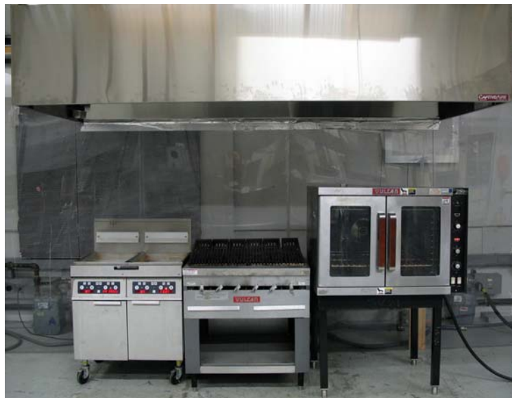
Figure 8. Fryer/Broiler/Convection Oven Appliance Line
