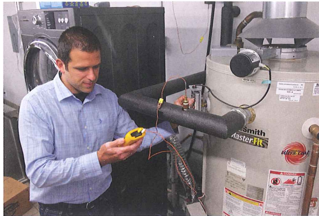
Monitoring hot water consumption will play a key role in the The Comprehensive Commercial Kitchen Equipment Retrofit Project.
